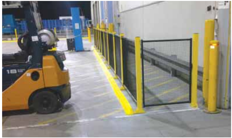
De-fence as pedestrian separation.
